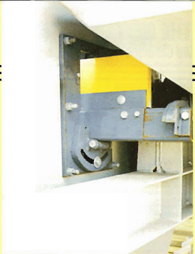
Model RLP and RFA Cleaners, with Flange Mounting Plates, installed on a conveyor discharge chute at Brunswick Pulp and Paper in Brunswick, Georgia.
